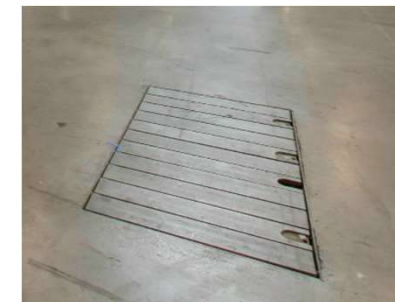
Technical duct on the floor
